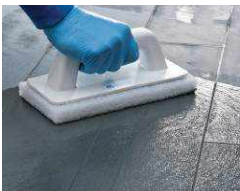
Cleaning the joints with a Scotch-Brite® pad (when the product is semi hardened)
