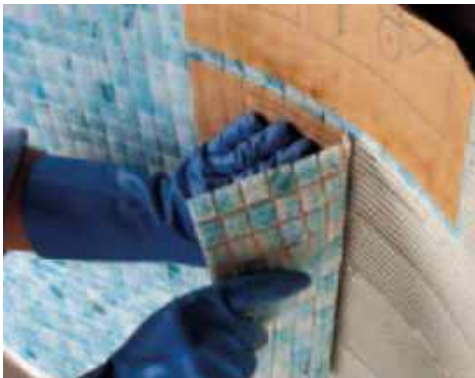
Glass mosaic 2x2 cm installation in a swimming pool with Adesilex P10 mixed with Isolastic diluted 1:1
